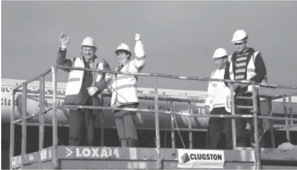
Lucie Calow, head teacher of the Granta school, tops out the new building with director of education for South Cambridgeshire, Andrew Barter. A Cambridge Evening News reporter and a construction worker look on.
